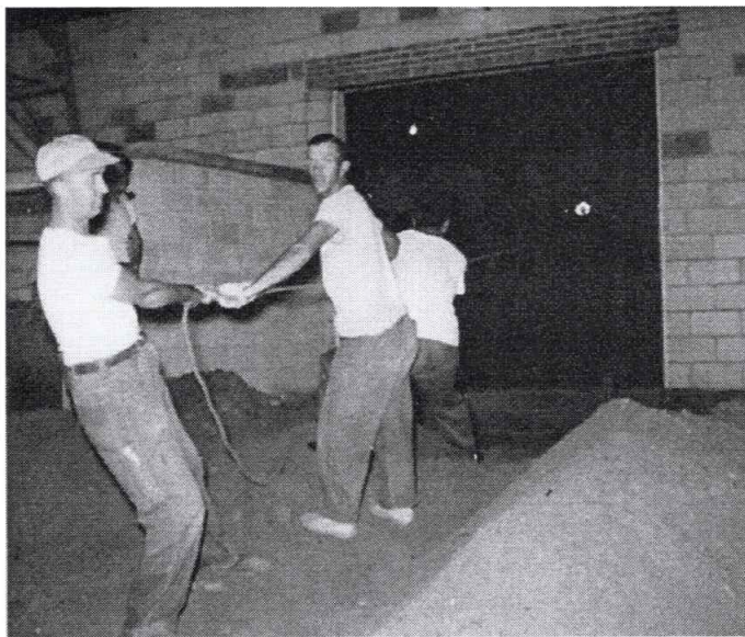
Members installing a 1000 gallon heating oil tank near the rear overhead door. Left: Horace McCurdy, (Behind Horace), Clifford "Pete" Litle, Ed Lamb, (-?-)
